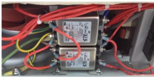
Two EMC filters fitted, Heater & Microwave*
