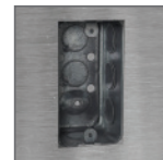
TA-62F Empty Junction Box
