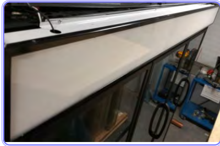
Display Slides out to access Wireway
